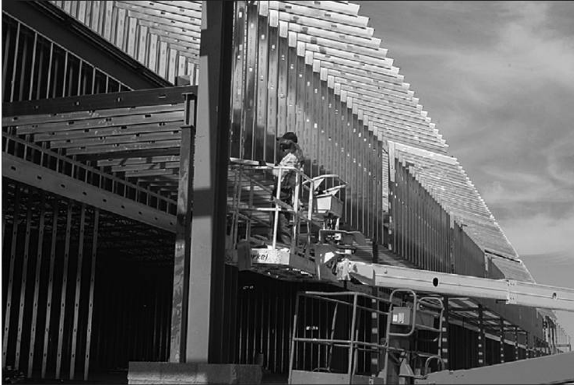
Staff photo by Jason Smith Construction worker Jorge Acosta places exterior metal studs on the outside of the new Coach store at the Tanger Outlet Center on Tuesday. The expansion is expected to be complete early next year.
